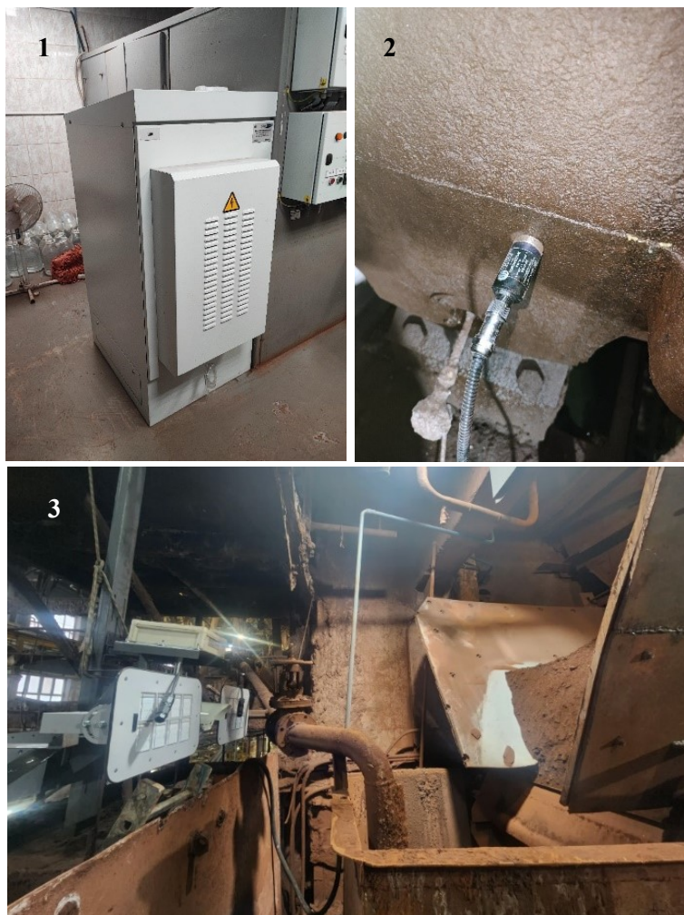
Figure 2. Data cabinet (1), vibration sensor (2) and machine vision unit (3).
